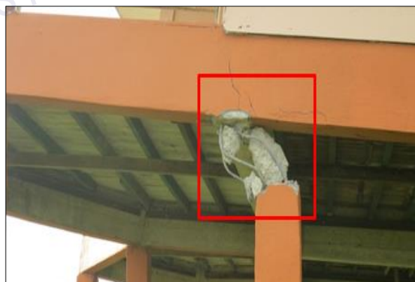
Figure 1.1: RC beam-column joint damage caused by Ranau earthquake
