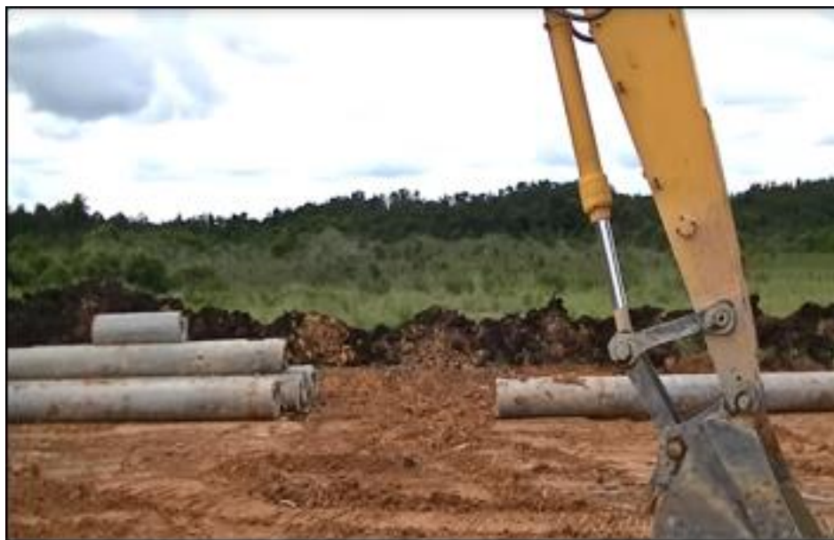
Figure 1.2: Removal and replacement method of peat at Sedenak Factory Park Project, Sedenak, Johor, Malaysia.
