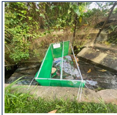
Figure 4. Installation of the Portable Rubbish Cage Trap in the drainage system in Taman Universiti Johor Bahru
