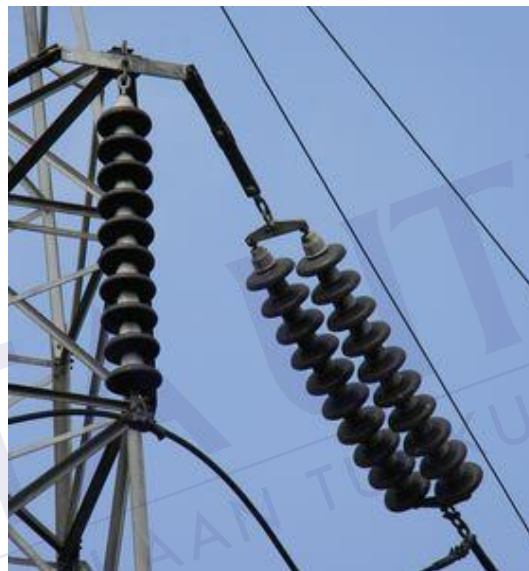
Figure 1.1 Polymeric outdoor insulators
