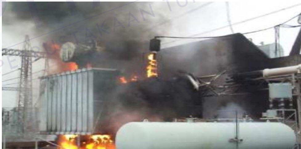
Figure 1.1: Damage of transformer at TNB substation due to lightning strike
