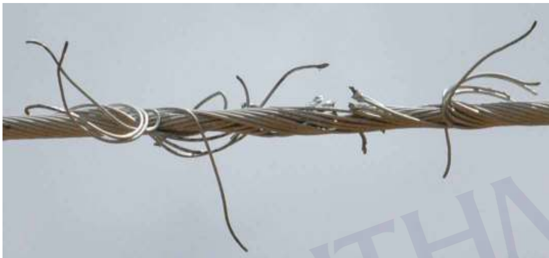
Figure 2.6 : Conductor damage due to vandalism resulting in broken strands and exposure of core.
