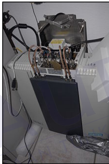
Figure 2.1: Base Transceiver Station (BTS)
