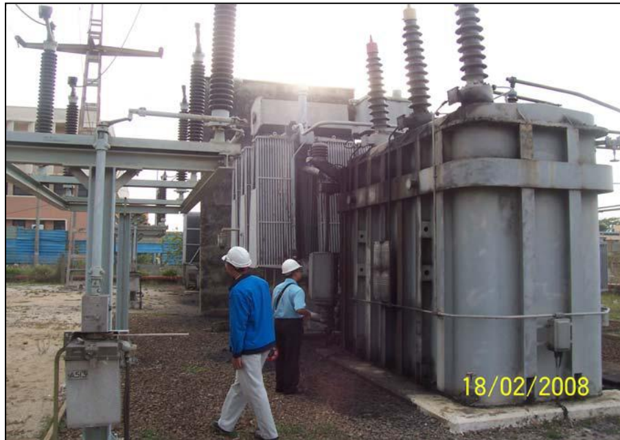
Figure 1.1 One of transformer owned by Tenaga Nasional Berhad
