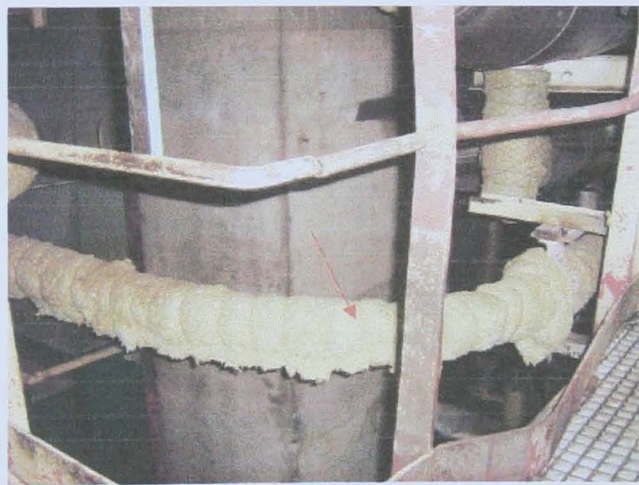
Figure 1.1: Insulated steam trap bypass tube in actual process.
