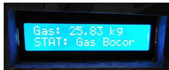
Figure 5(b). : LCD screen displays the LPG mass and gas leakage status
