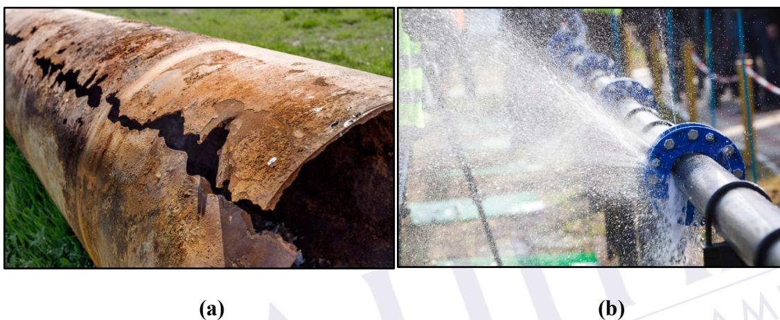
Figure 1.1: Sample pipeline problems (a) Corrosion on pipe; (b) Pipe burst
